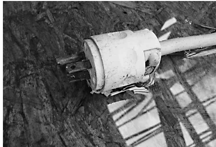
Be alert to electrical equipment that could be energized and in contact with water, creating a serious danger of electrocution.
